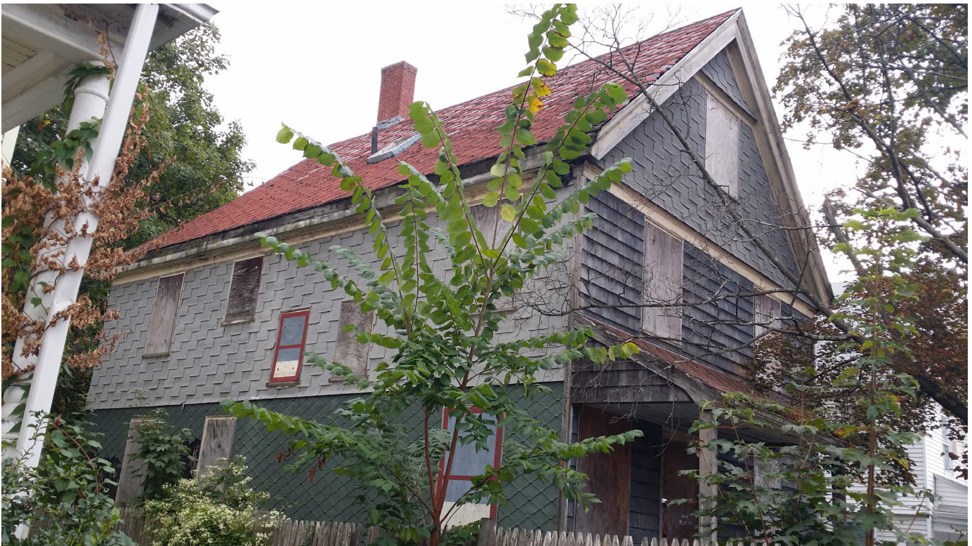
556 Park Street first appeared on the tax-delinquency rolls in 1999, but was not foreclosed upon until 2011. It remained under appeal until 2014, but is currently in the first stages of assessment, pre-disposition.
